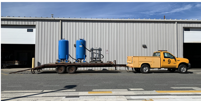
Weston implemented a mobile PFAS treatment system used to treat water pumped from the fuel farm containment system prior to discharge at a municipal airport in Massachusetts.
