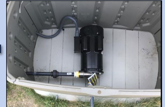
Groundwater Transfer Pump
