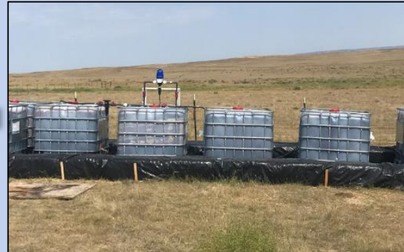
Sodium Permanganate Totes
