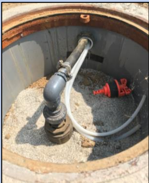
Injection Well Cap
