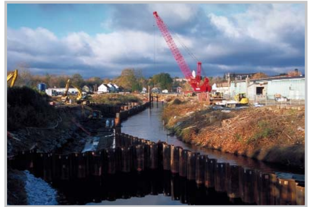
WESTON established an extensive system of dry areas and temporary dams to divert the Housatonic River and remediate 95,000 cubic yards of PCB-contaminated sediment.
