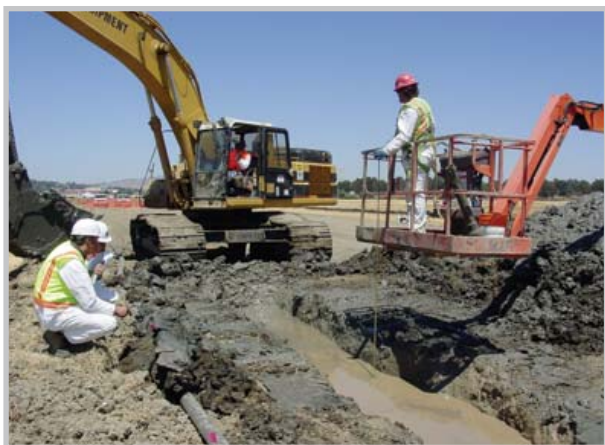
As part of the overall island development, WESTON is remediating a 72-acre former landfill and preparing it for final closure.
