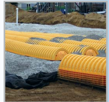
Stormwater is managed on site with a subsurface drainage system.
