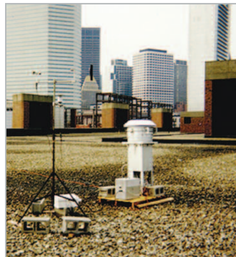
To maintain compliance, WESTON harnesses proven technologies such as this Rooftop Pollutant and Meteorological Monitoring Station
