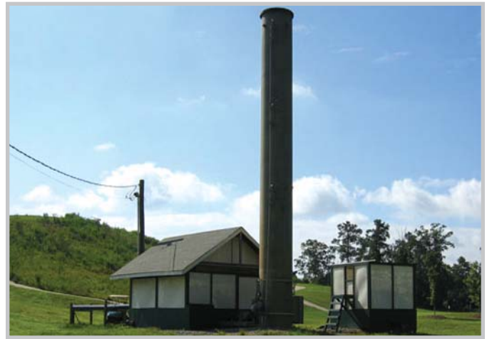
▼ Gas collection and control systems are designed to integrate with the surrounding environment.
