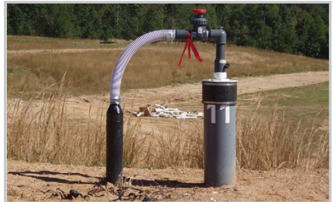
▼ WESTON performs wellfield balancing of gas collection and control systems.
