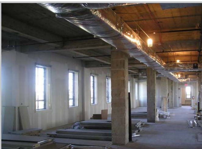
Enhanced Use Leasing allows private developers to assist the DOD in rejuvenating unused buildings and earn the economic rewards from leasing the property.
