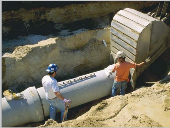
WESTON provides a full complement of consulting, engineering, construction and operations services
