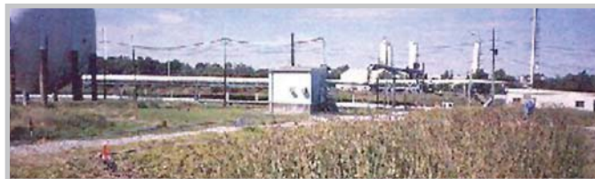
Constructed wetlands treat petroleum residuals in refinery waste, meeting strict permit discharge limits
