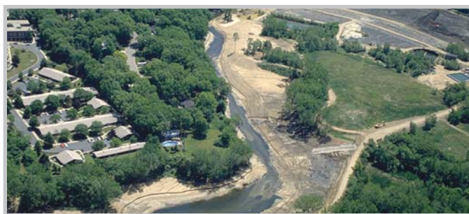
Following cleanup, pools, riffles, and meanders are created as part of the restoration design.
