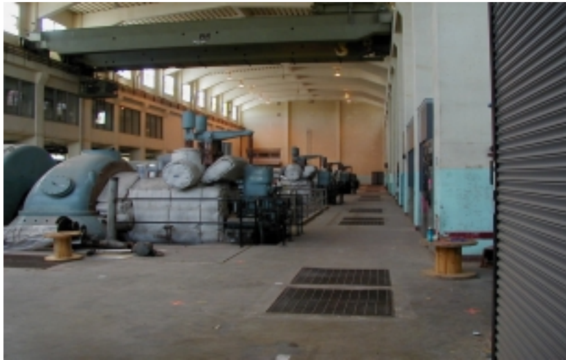
Seaholm Power Plant Turbine Hall
